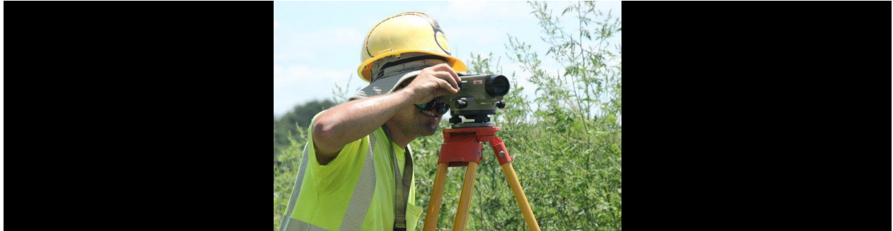
Nathan Knorr does survey work for the Fort Hamer Bridge project Thursday. JAMES A. JONES JR./Bradenton Herald
