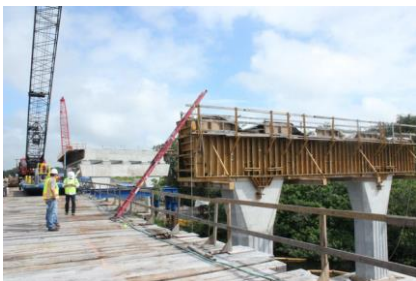
Forms used to pour concrete for a set of piers for the Fort Hamer Bridge may soon be removed.
