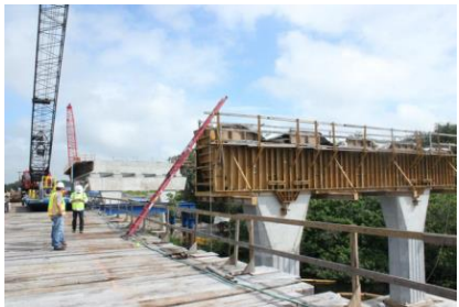
Three sets of piers have been poured for the new bridge over the Manatee River.
