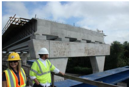
Concrete will be poured over these I-beams to provide the driving surface on the Fort Hamer Bridge.
