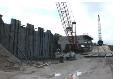
The ground around the northern terminus will need to dry out before cranes can position I-beams to connect it with the nearest set of piers.
