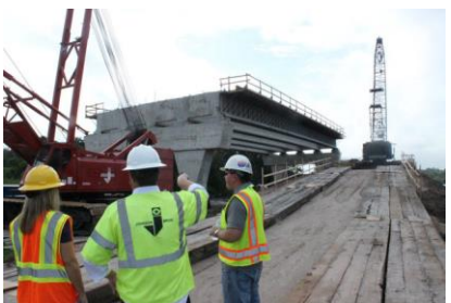
Two cranes are needed to lift and position the massive I-beams which provide the horizontal surface for the Fort Hamer Bridge.
