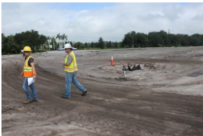
A new approach to the Fort Hamer Bridge is being developed and will help speed completion of the project.
