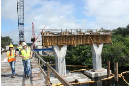
Trudy Gerena, Tom Charles, and Justin Hogan walk on a temporary bridge used for construction of the Fort Hamer Bridge. To the right is the first set of piers with footers in the water of the Manatee River.
