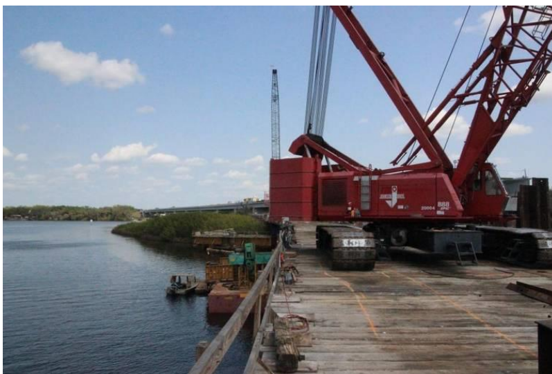
A crane is shown working from the construction trestle of the Fort Hamer Bridge near the south shore of the Manatee River in March. James A. Jones Jr. Herald file photo.
